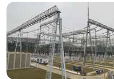
Electricity power inspection
